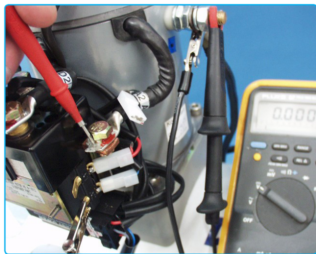
Checking voltage on A2 with ground to blue jumper attached and IPC wire disconnected.
