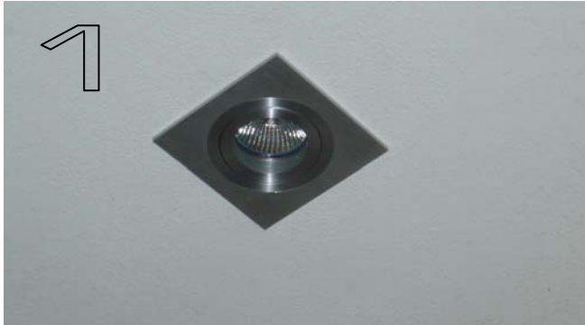
1 Spot Light with lamp requiring change-out
